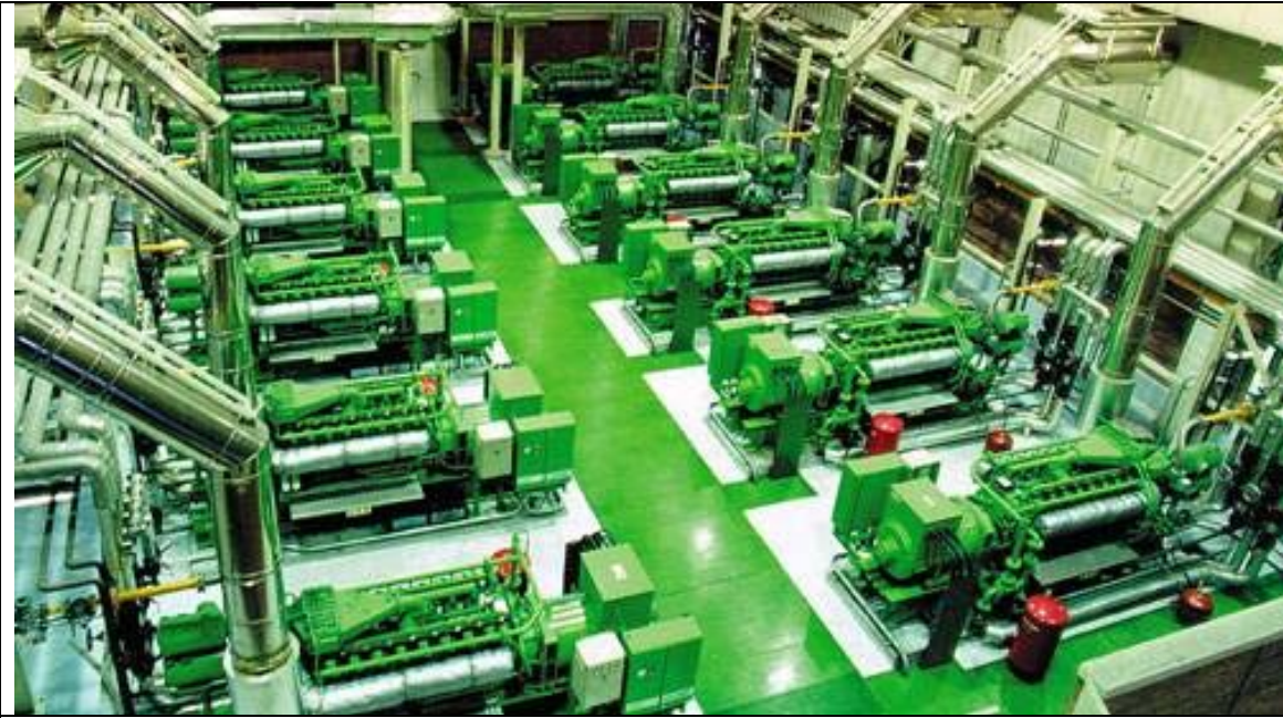
Figure 3-5: Conventional Internal Combustion gensets.
